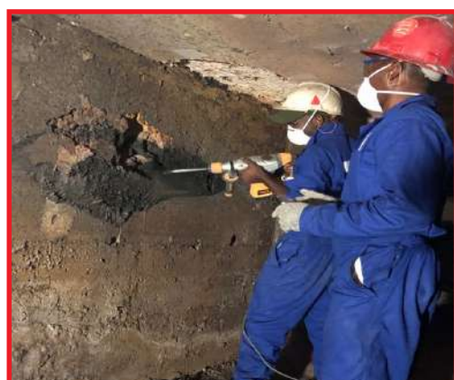
MORUPULE B AIR DUCT BURNER REPAIR (CUTTING TO SPOIL THE SUTE CAUSED BY SLAG)
